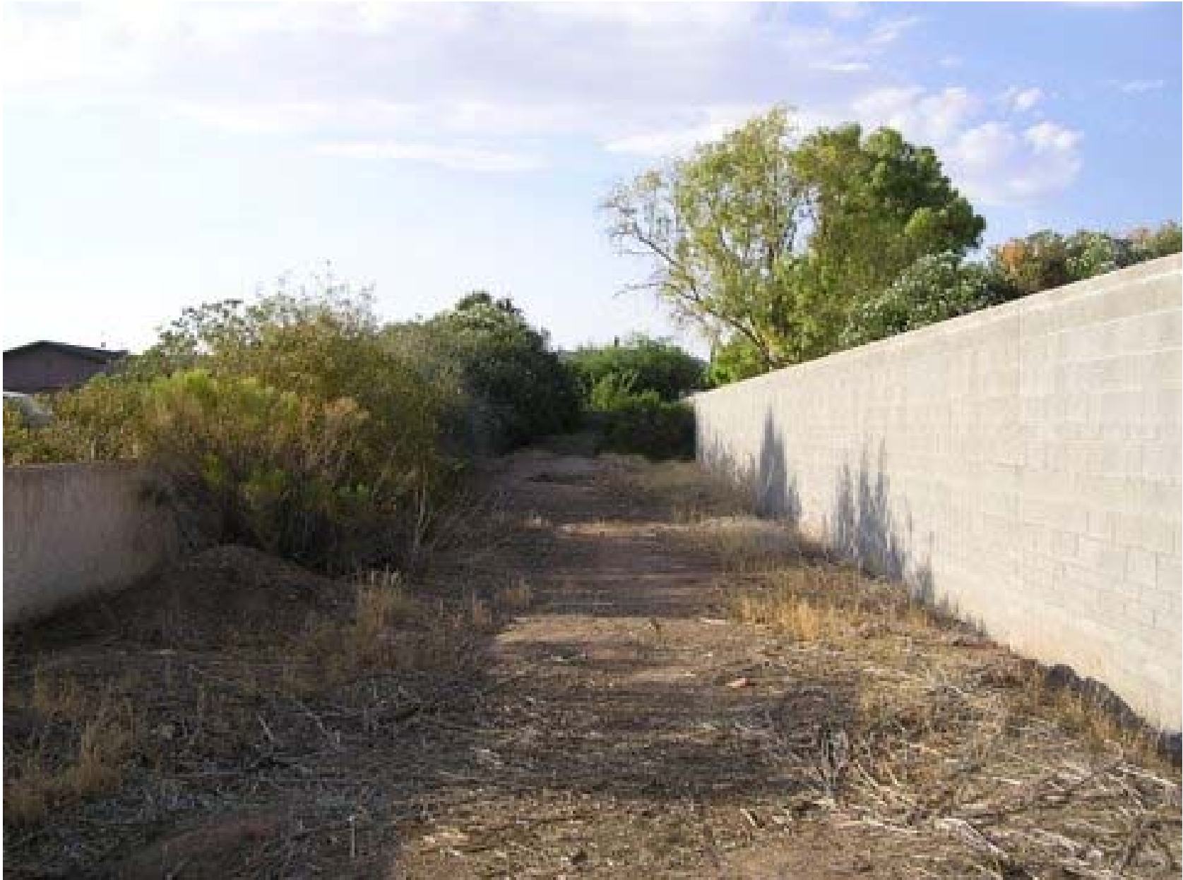
Residential Wall on Alley Side Before Tagging Near 32 nd Street/Indian School Road
